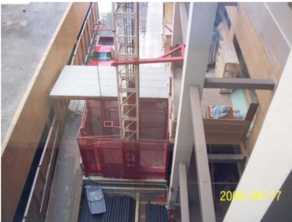
Figure 7 - Material Hoist/Loading Dock
